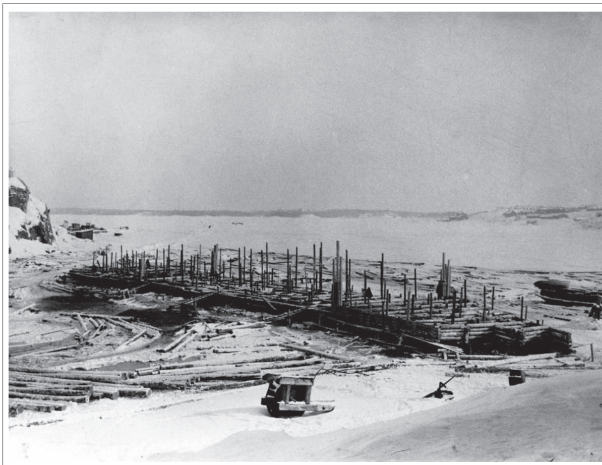
Fig. 1. The larger log-barrier embankment under construction, 17 February 1917, at the mouth of Tykistölahti Bay (Helsinki City Museum).
